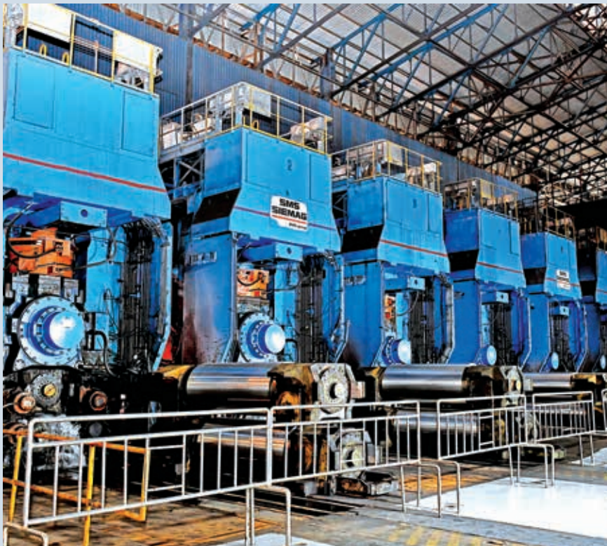
Thin slab caster and rolling facility at Jamshedpur Steel Works
